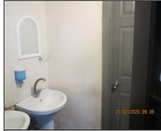
Photo of the sanitary facilities SANITARY FACILITY.JPG
